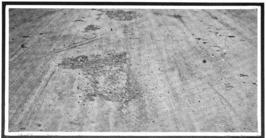
Where a calk wound has allowed water to penetrate, causing destruction of the road surface
